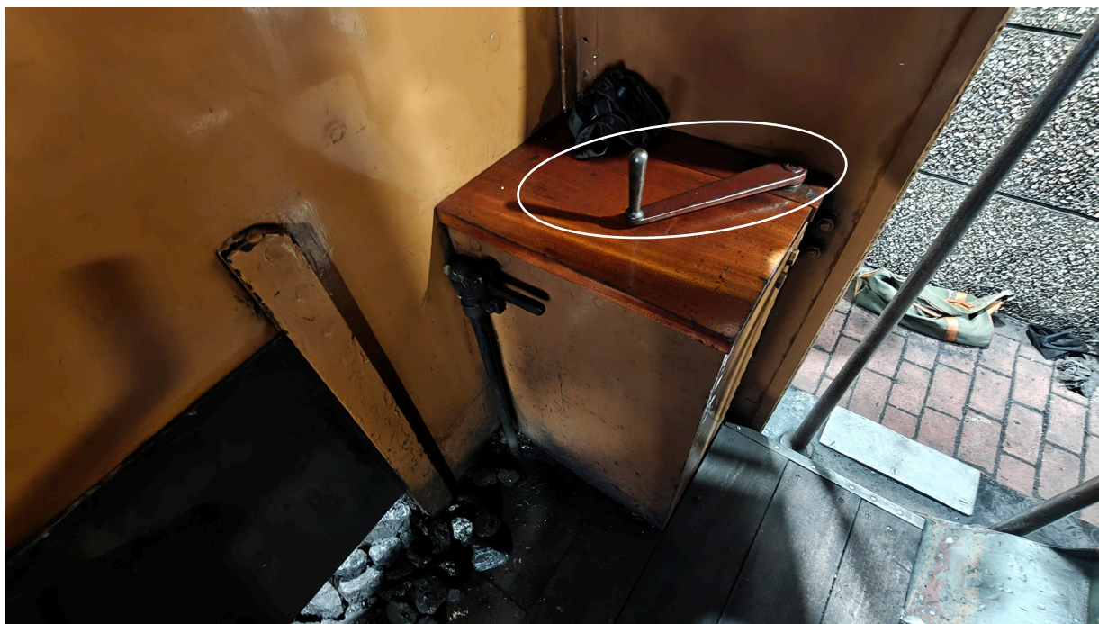
Figure 7: Drain cock operating handle on Fenchurch.
