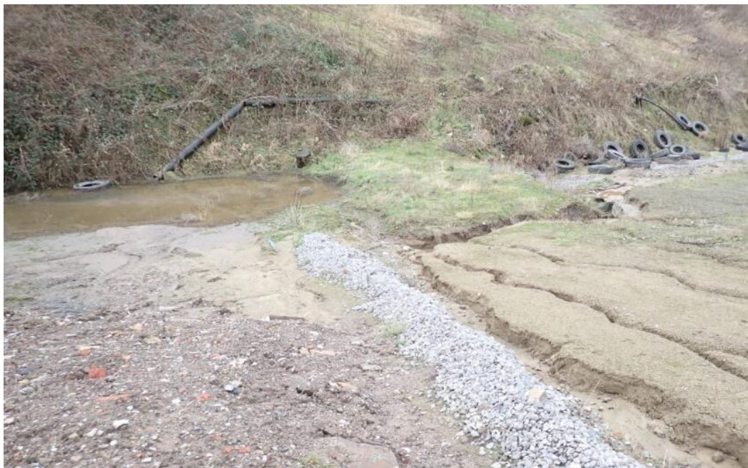
(Photo 9 – Pool of leachate/contaminated surface water where cell 3a and cell 5a meet)
