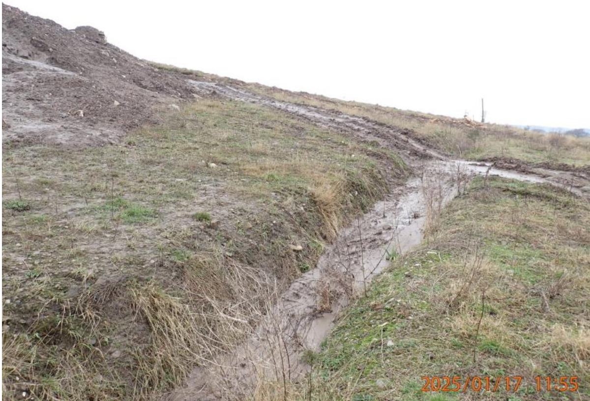
(Photo 13 – showing waste stacked on the cap running down to the sites road before entering the surface water management system)
