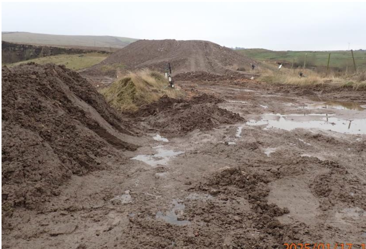
(Photo 2 Waste observed from a distance (not the material on the left) at the top of cell 4-5a – eye level)
