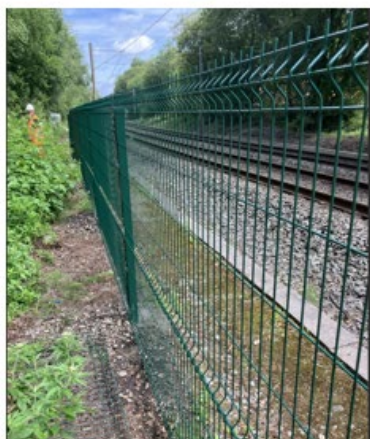
Lineside Security Fencing
