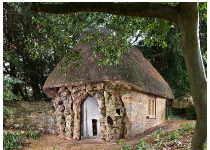
Dr Jenner's Hut in Gloucestershire, birthplace of vaccination, requires urgent repairs to secure its future and was added to the 2025 Heritage at Risk Register.
