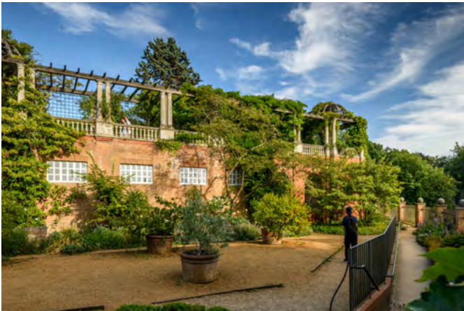
The Grade II* listed Hill Garden Pergola, a popular structure on the west side of Hampstead Heath, is starting to show its age and was added to the 2025 Heritage at Risk Register.
