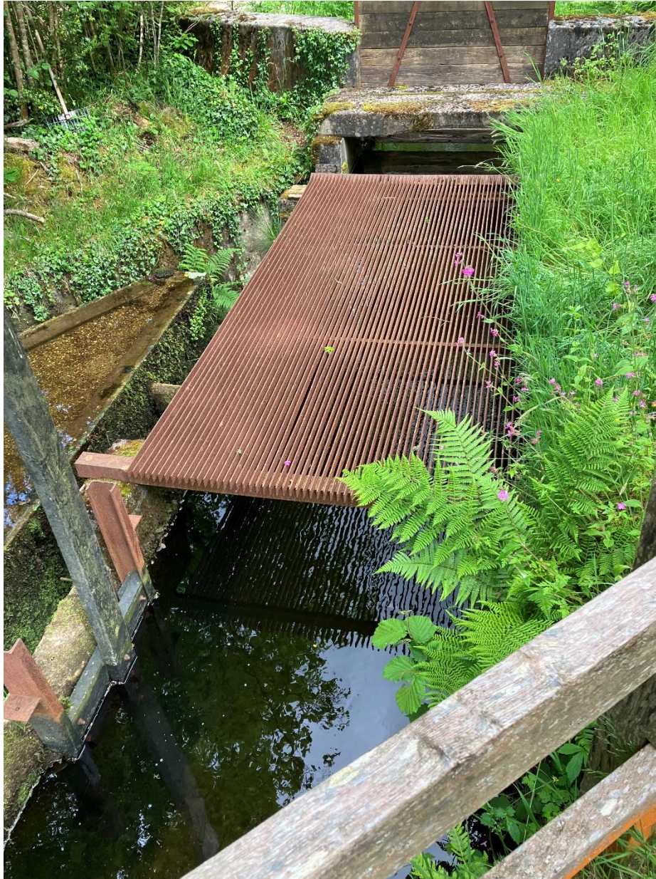
Fig 2.0 Kelt screen and intake sluice.
