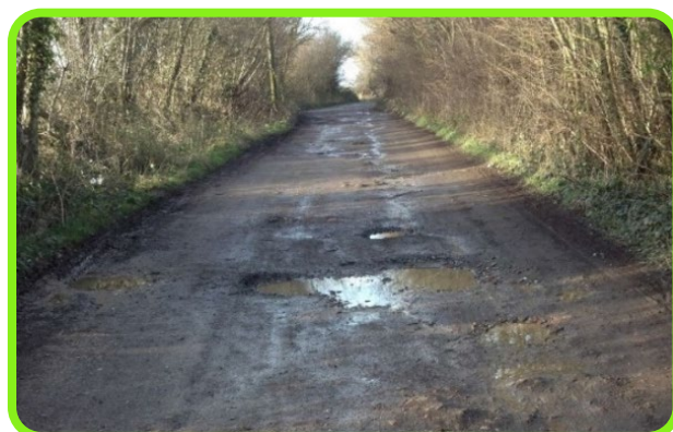
Figure 4: Poor quality of the carriageway surface prior to resurfacing.
