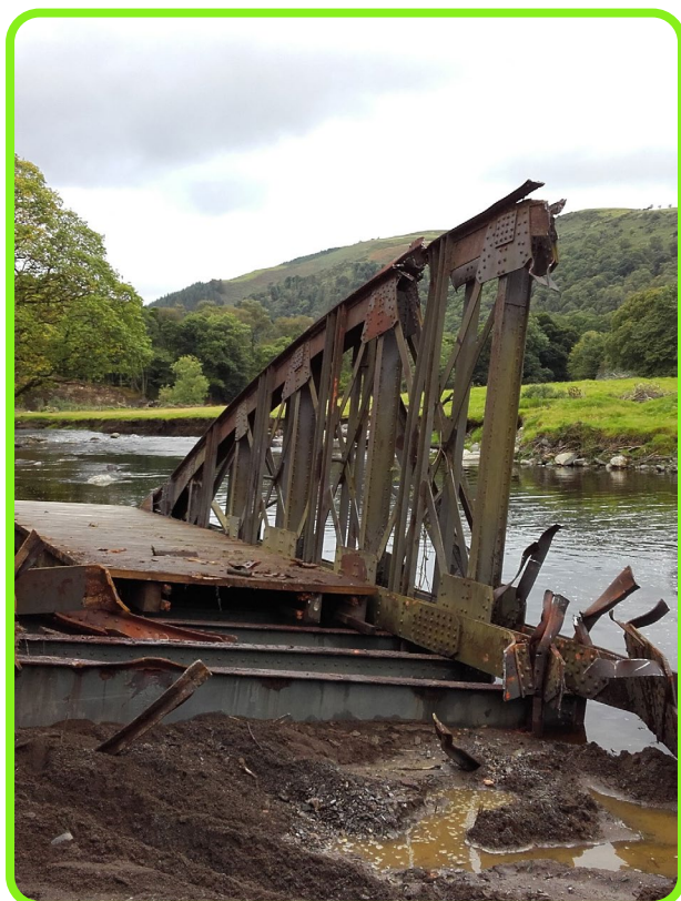
Figure 3: Damage to the Keswick to Threlkeld Trail from Storm Desmond.
