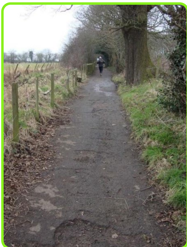
Figure 3: Condition of the path prior to resurfacing.
