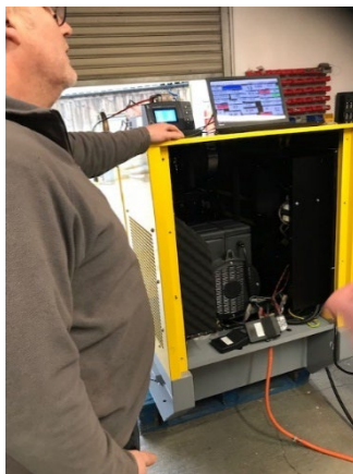
Figure 4. Initial installation and testing of new HGE ECU
