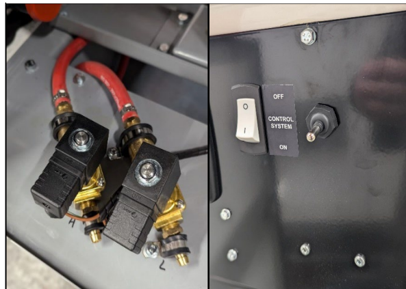
Figure 19 H2 and LPG Shut-down valves and fuel changeover switch
