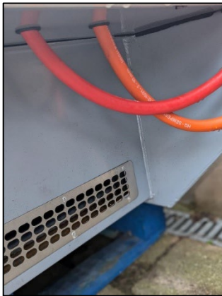
Figure 18. H2 feed-pipe red, LPG pipe
