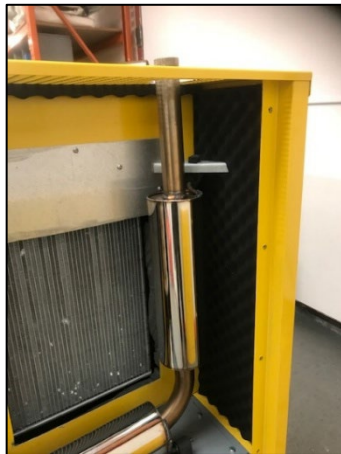
Figure 8 Exhaust installed in genset
