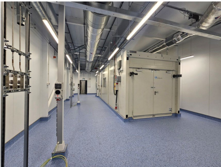
Figure 40: MCL in completed lab
