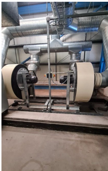
Figure 7: Load balanced extraction fans
