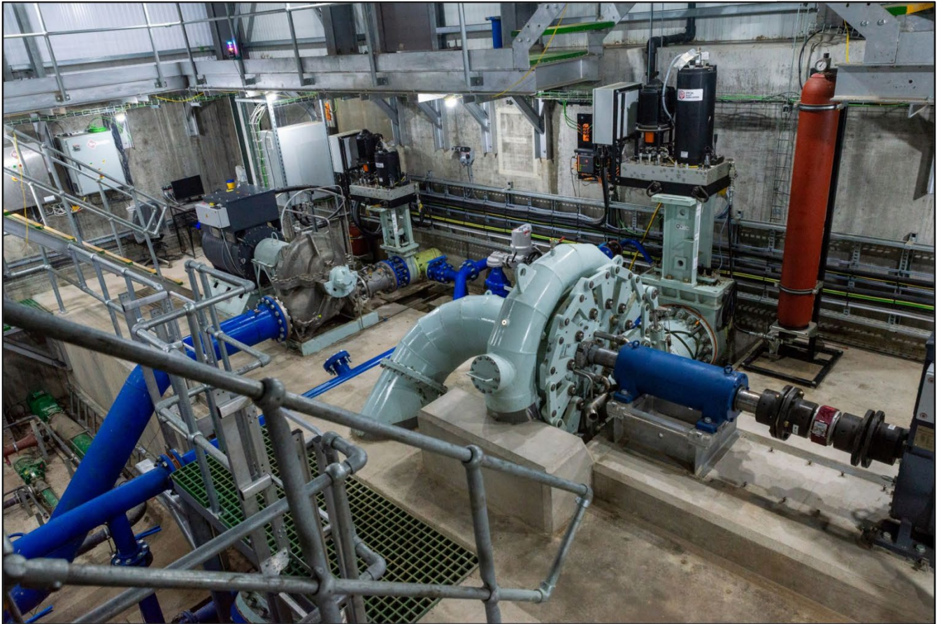
Figure 21 Powerhouse views of turbine pump and MIVs and towards FMS
