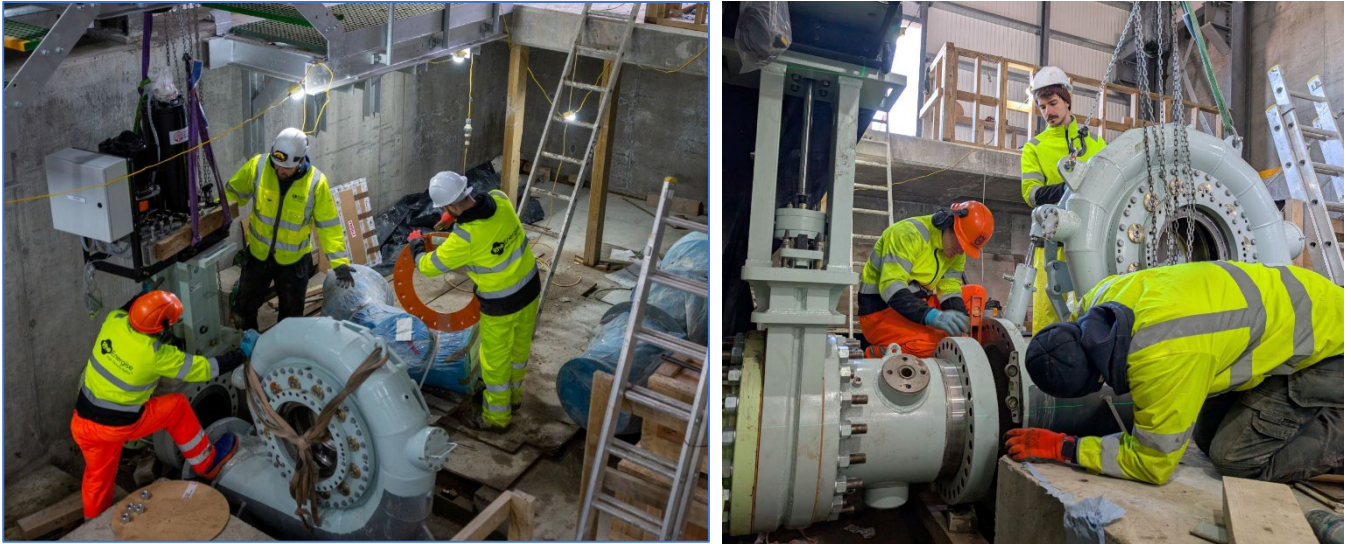
Figure 20 Positioning of turbine and main inlet valve
