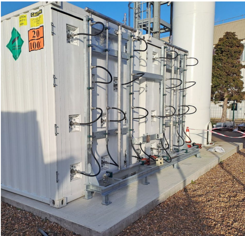
Figure 4: Containerised air stores
