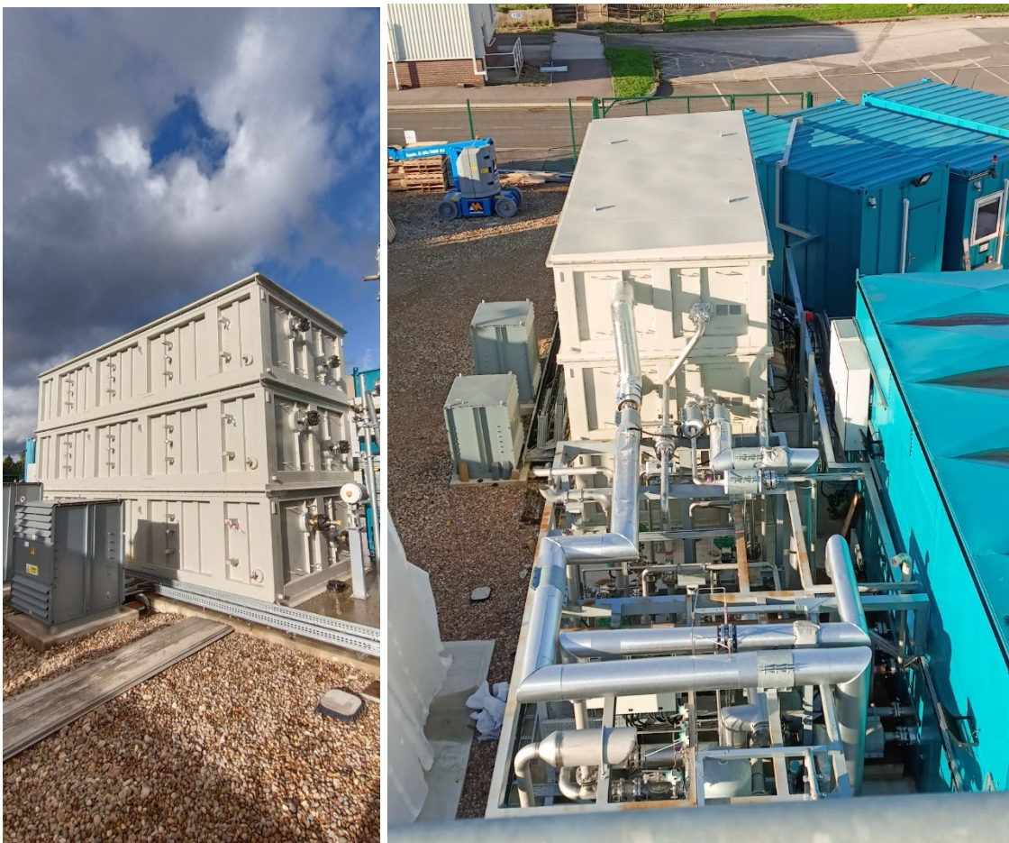
Figure 5: Views of the thermal store from the side and from above
