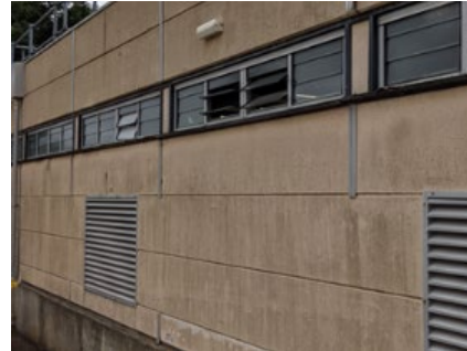
Figure 4: Example of RAAC in walls
