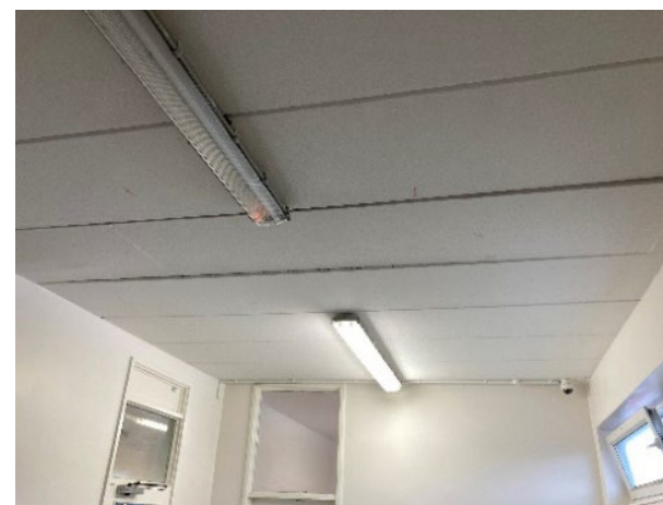
Figure 11: Example of deflected RAAC panel
