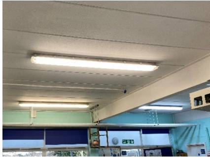
Figure 3: Example of RAAC in flat roofs/floors
