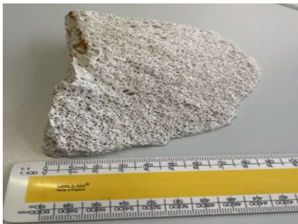
Figure 6: Aerated appearance of RAAC
