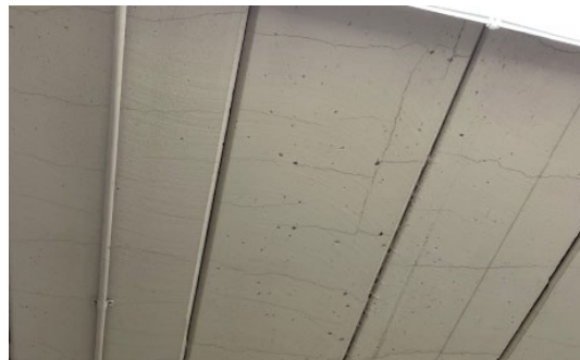
Figure 7: Underside of a cracked RAAC panel
