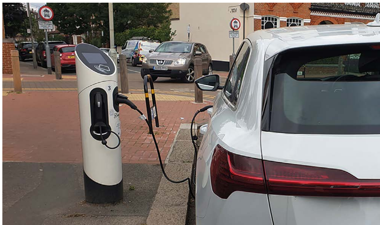
An EV chargepoint plugged into an EV
