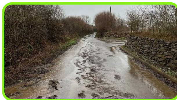
Figure 14-18: Country lane with poor drainage – South Hams, Devon.
