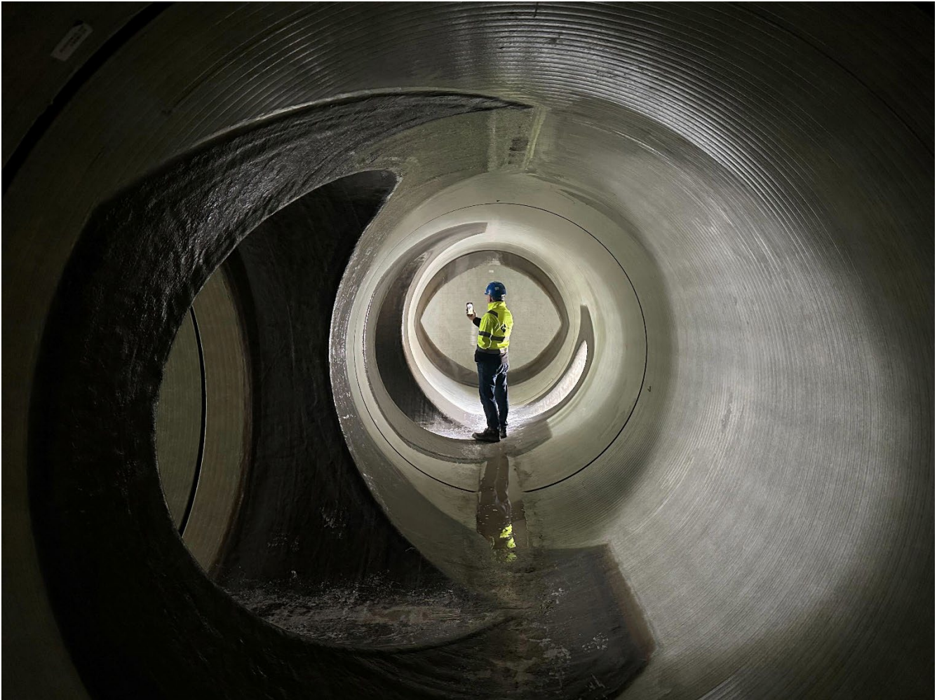
Figure 1: In the upper reservoir at RheEnergy's High-Density Hydro® energy storage facility in Devon, UK, supported by DESNZ funding of more than £9 million through the Longer Duration Energy Storage Stream 2 programme.
