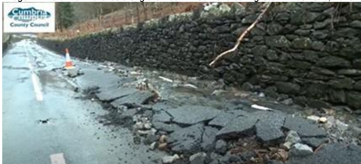
Image 17. Earthwork failures along the A591 in Cumbria during Storm Desmond, 2015.
