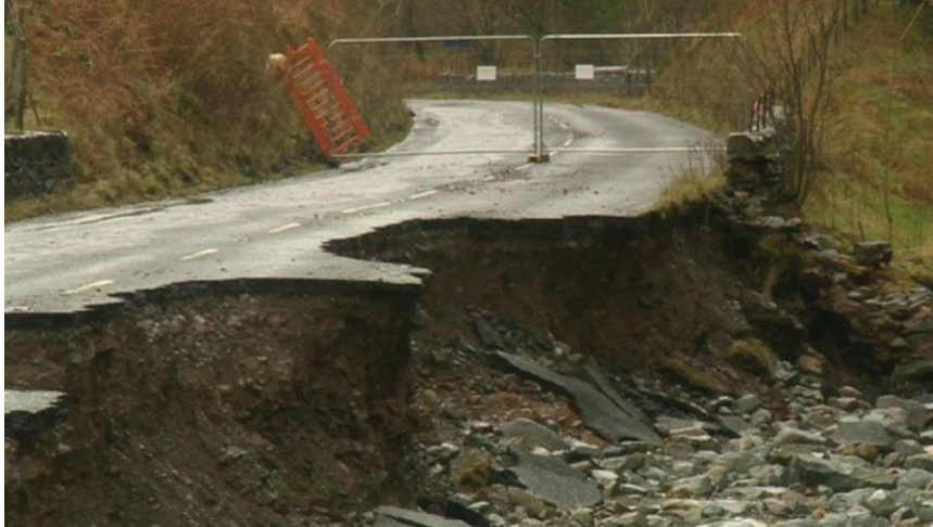
Image 4. Partially collapsed section of road on the A591 during Storm Desmond.
