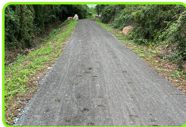
Figure 5: Damage caused to limestone dust surface by horse riders.
