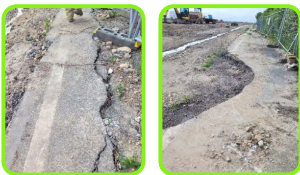
Figure 6: Poor surfacing on Wild Lane prior to upgrade.
