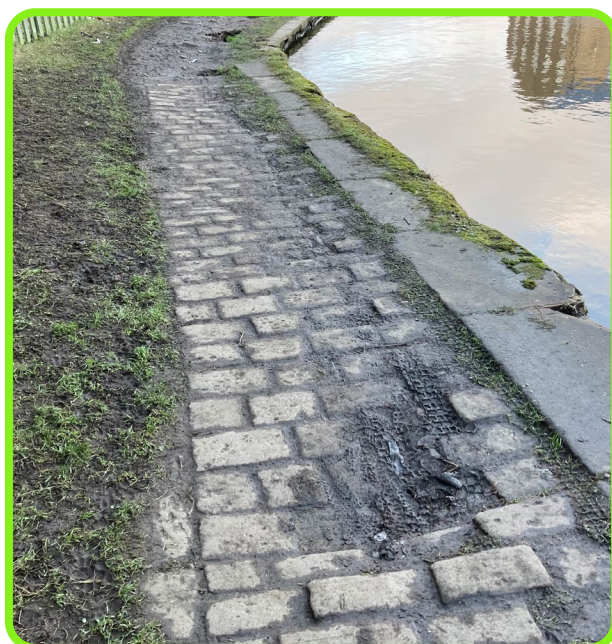
Figure 4: Stone setts before improvements.
