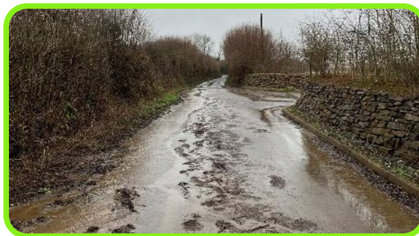
Figure 14-18: Country lane with poor drainage – South Hams, Devon.
