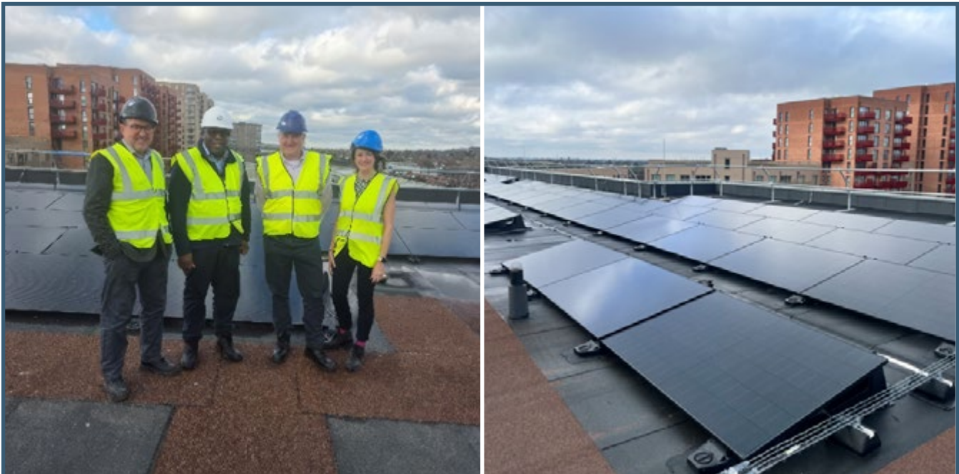
Solar panels installed on the roof of Harrow Crown Court
