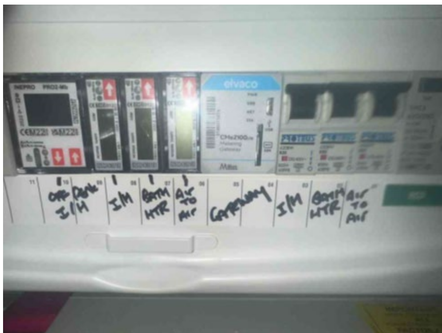
Figure 70: Photo from site showing submetering arrangement in newly installed distribution board 43 .
