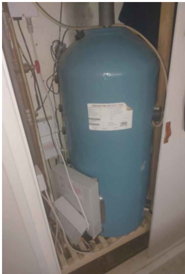
Figure 2: Photo from site showing micro-server attached to hot water cylinder
