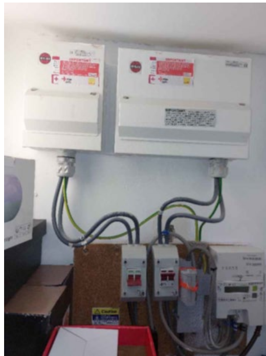
Figure 71: Photo from site showing separate distribution boards for off-peak heating (top left) and all other circuits (top right), each with isolator switch (bottom centre). Smart meter (bottom right) and DNO incoming fuse (between meter and isolator switches)
