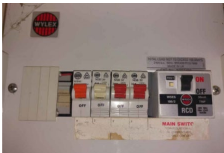
Figure 69: Photo from site showing distribution board with poor labelling of circuits
