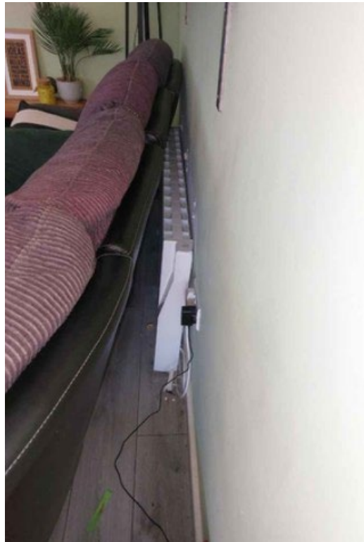
Figure 68: Photo from site showing permanent wall-mounted heater which appears to be plugged into a ring-main socket. An absence of dedicated heating circuits in this home's distribution board supports this conclusion.
