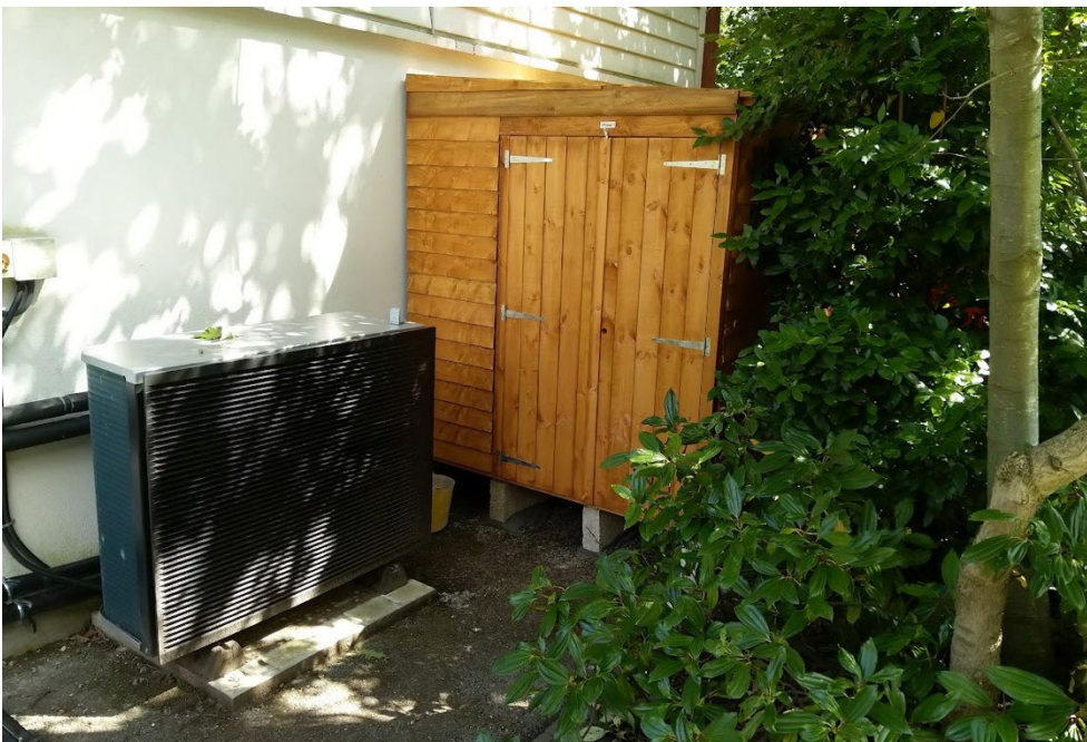
Figure 3: The Daikin heat pump alongside the shed constructed to house the TCS system.
