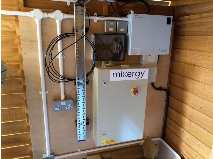
Figure 52: Electrical provision in external shed of the dwelling.
