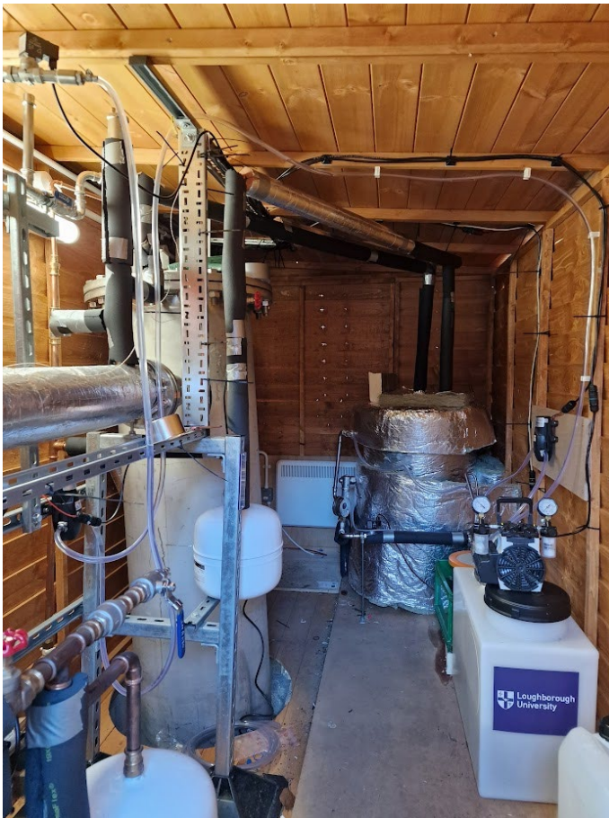
Figure 56: Completed TCS Gen 2 system at the dwelling.
