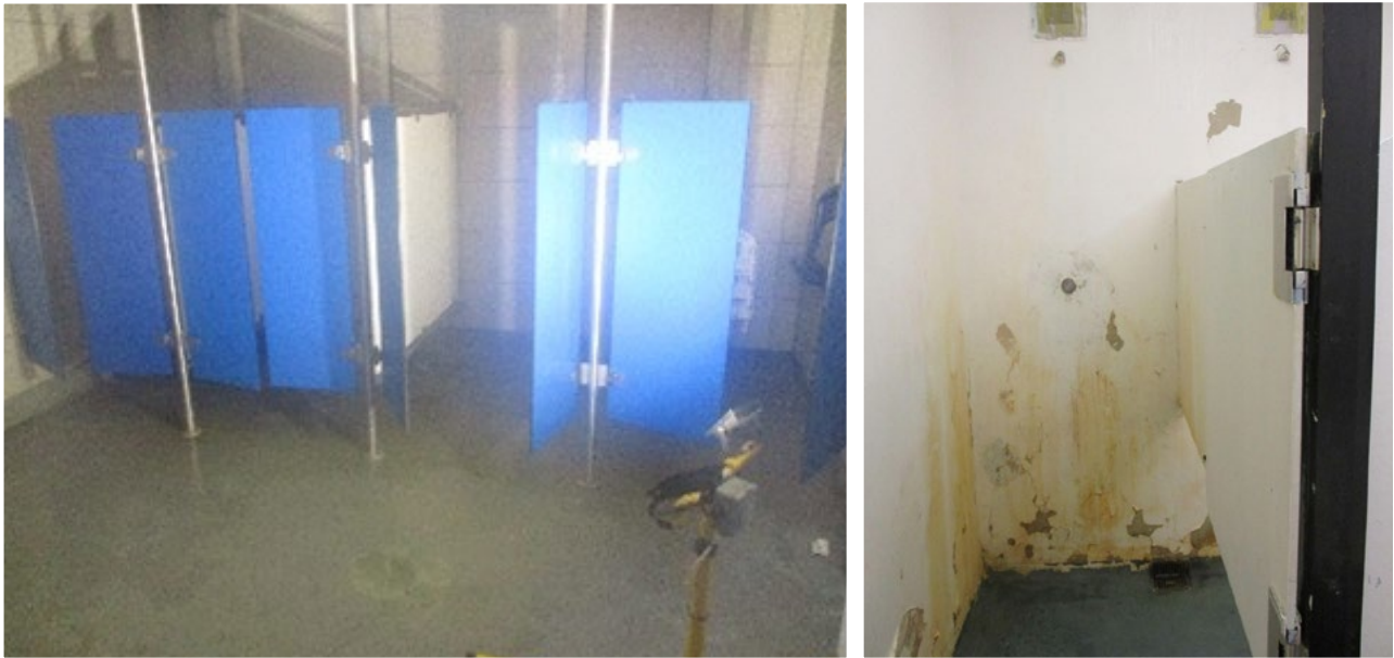
Left to right: temporary lighting in showers at Guys Marsh and damaged shower in Birmingham
