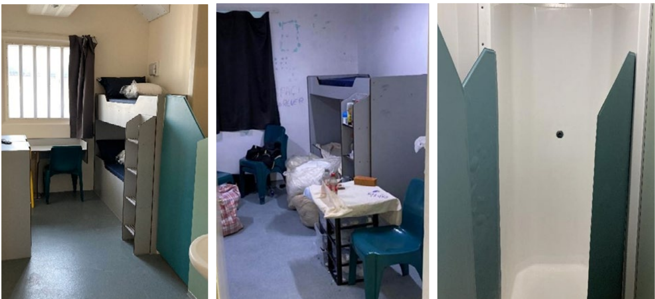
Left to right: refurbished cell, the cell at the previous inspection and a refurbished shower at Harmondsworth
