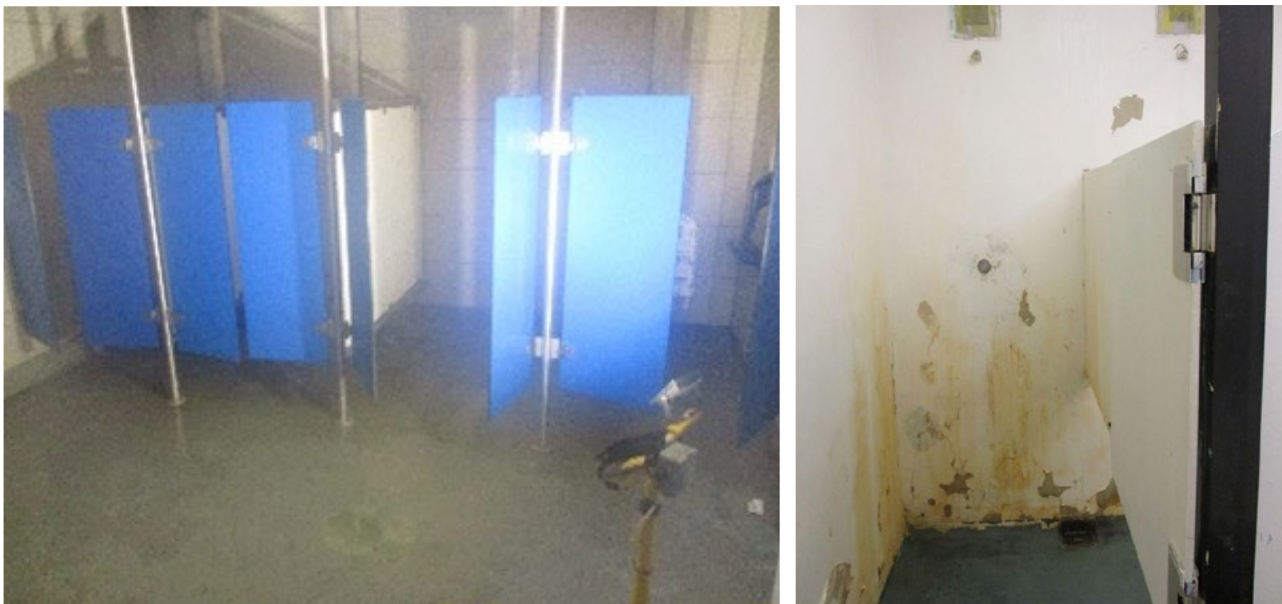
Left to right: temporary lighting in showers at Guys Marsh and damaged shower in Birmingham
