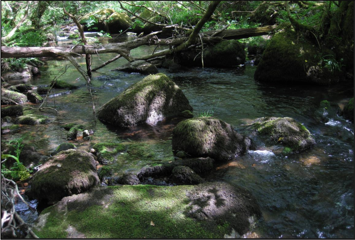
Image 1: Water through the notch leaving the rest of the weir exposed (May 2018)
