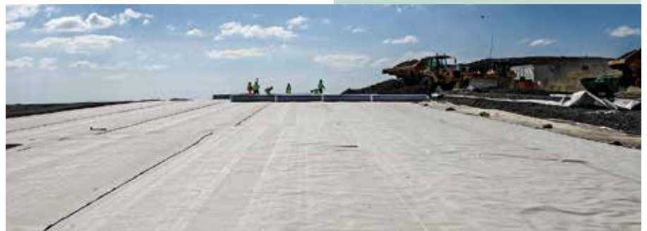
The liner is laid during the drier months due to its efficient absorption of water
