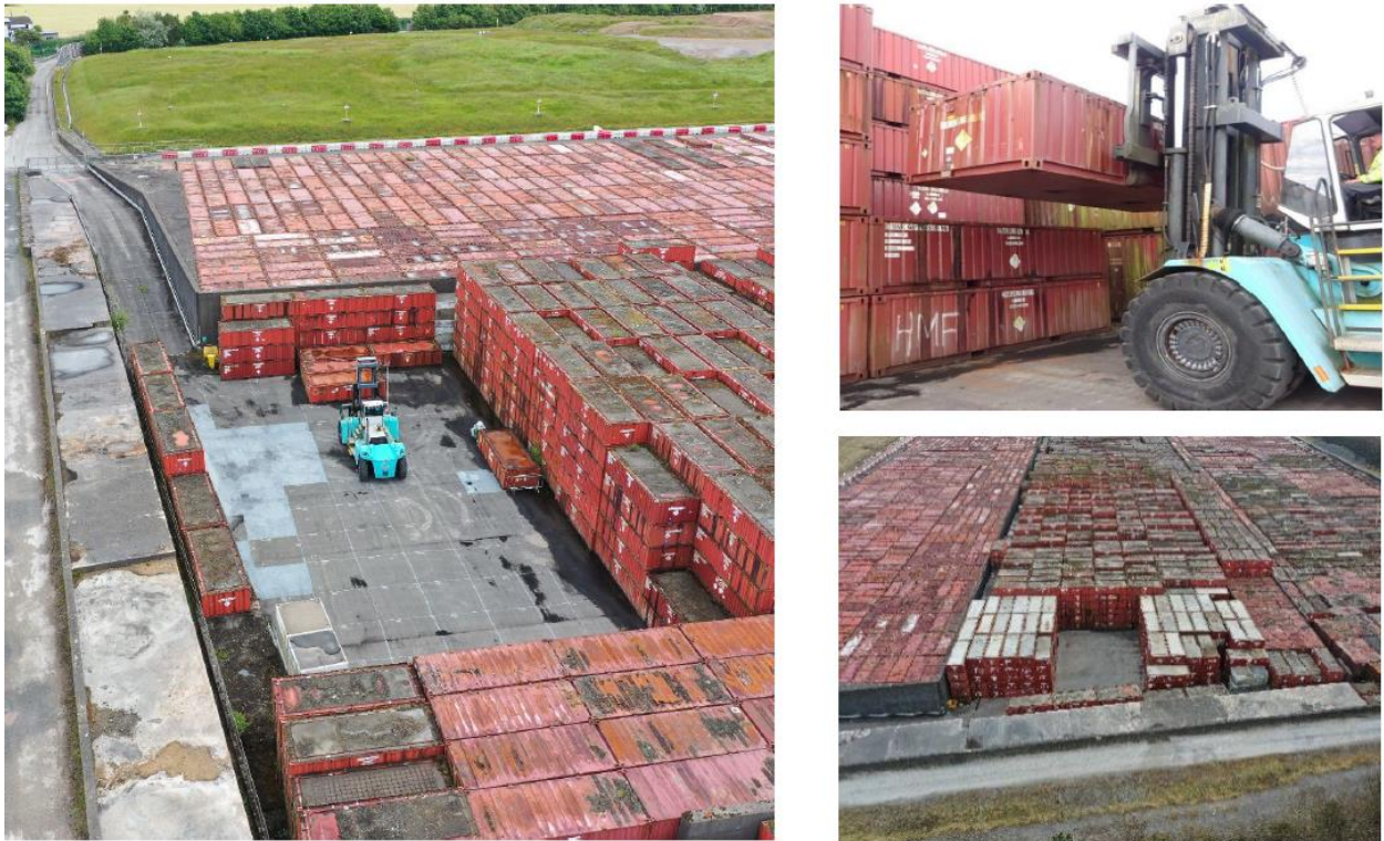
Figure 5.3: Progress in Vault 8 Remaining Disposal Volume Utilisation Ahead of Final Capping (Photographs capture different stages of work in progress)
