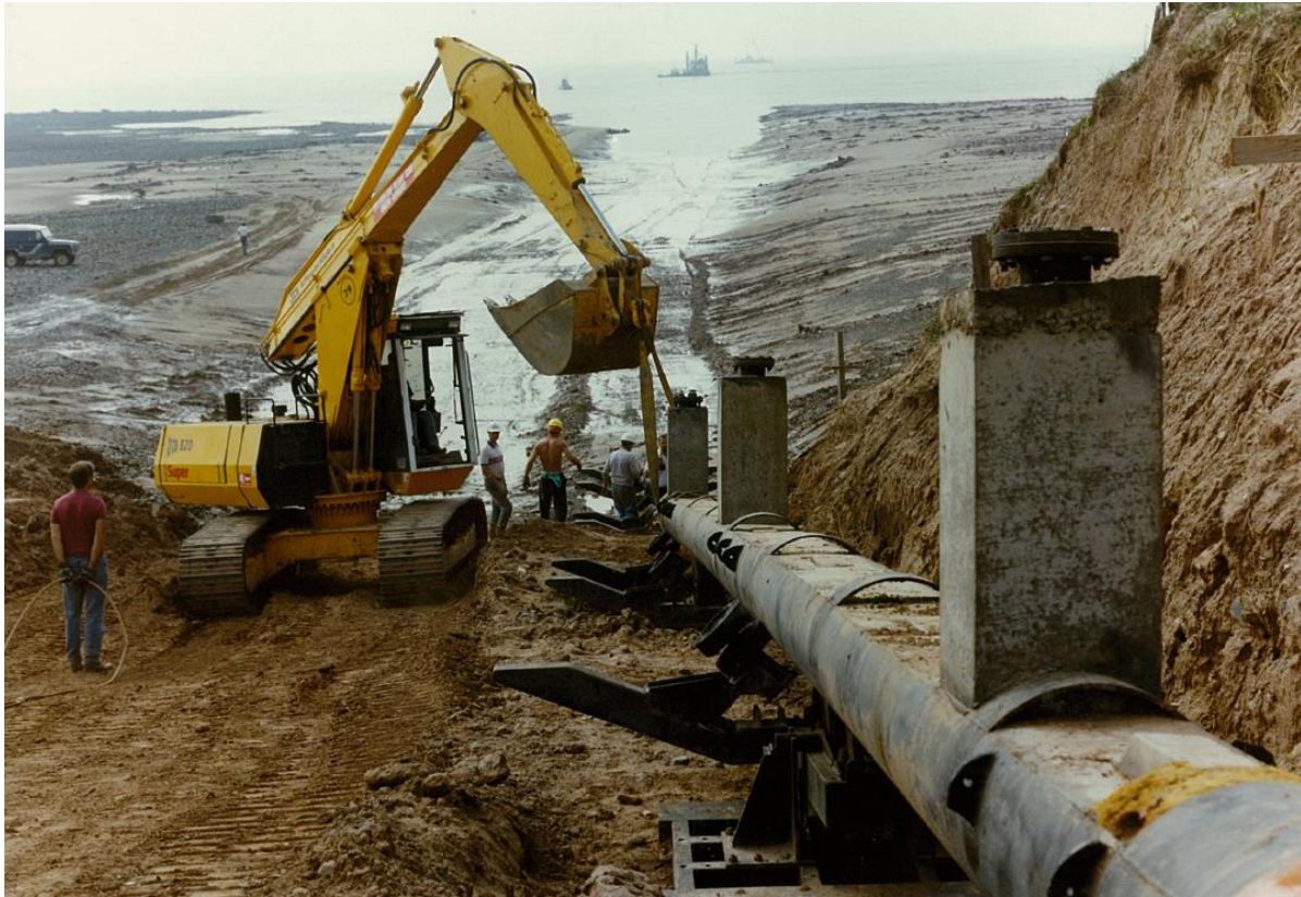
Figure 2.12: Photograph of marine diffusers prior to emplacement during the construction of the Marine Pipeline
