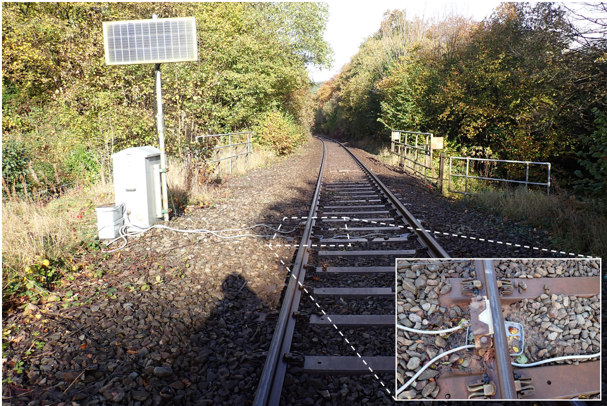
Figure 52: Non-functioning Talerddig 1 TGA; note the plastic lid under the rail which has collected small sand particles from the traction gel (likely when they are washed off the rail by rain).
