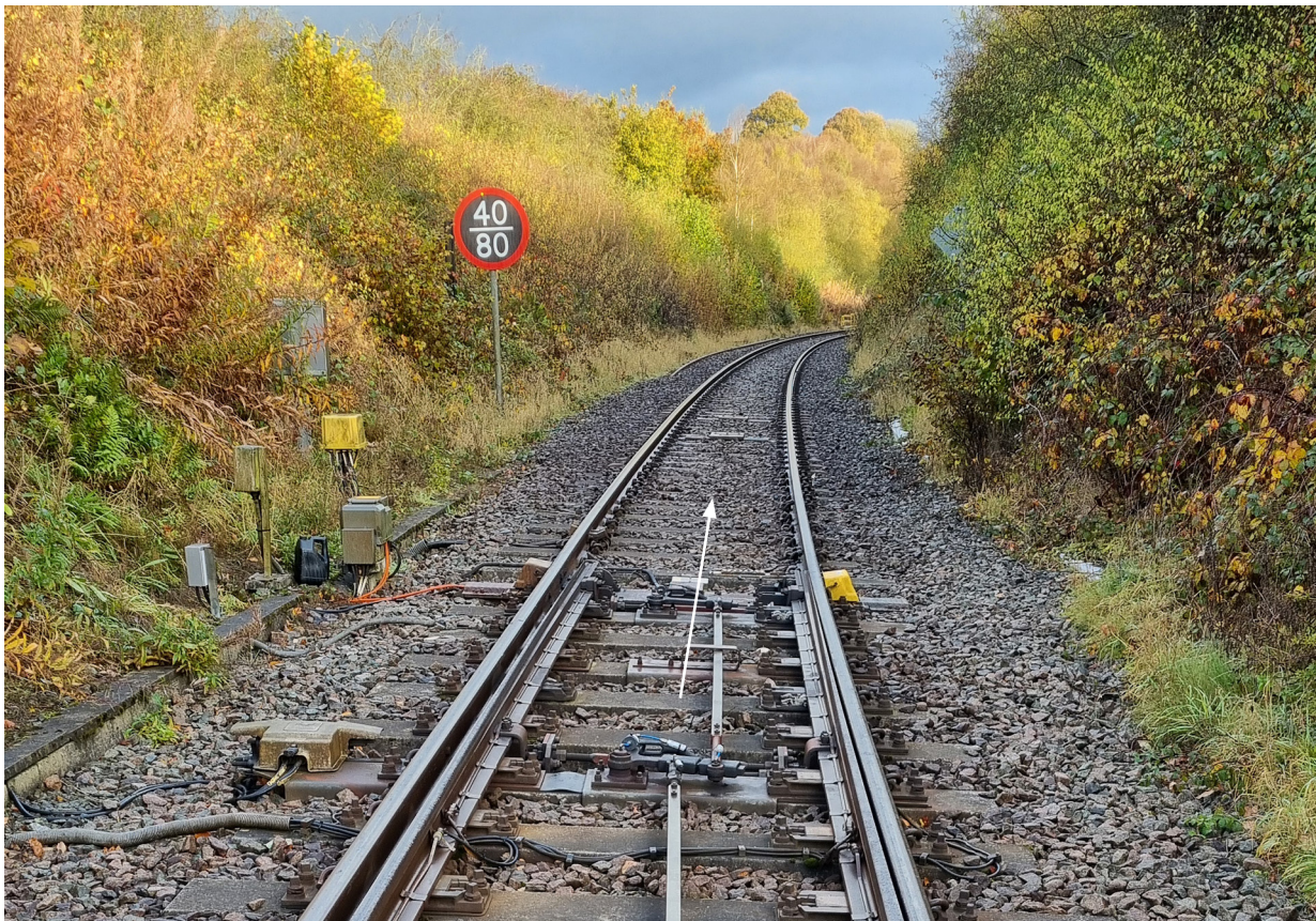
Figure 50: Lineside vegetation, in vicinity of the exit points of Talerddig loop at around 09:20 on 22/10/24 (the collision location is approximately 900 m away).
