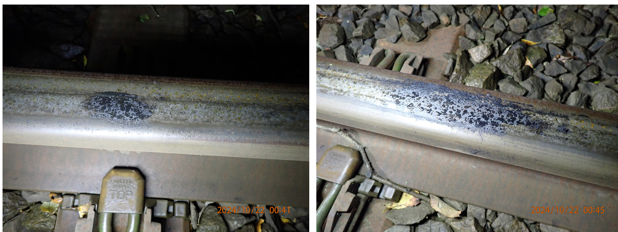
Figure 24: Example of visible contamination observed on the railhead between the collision location and Talerddig loop at around 00:45 hours on 22/10/2024.
