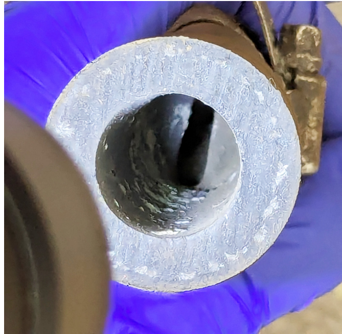
Figure C9: After cutting the hose near the hose clamp, the restriction in the sand hose can be seen, accounting for approximately a 60% loss in cross-sectional area of the sand hose.
