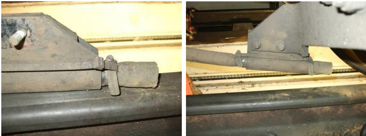
Figure C10: Extract from RSSB Sander maintenance good practice guide showing poor practice with hose clamps (courtesy of RSSB).
