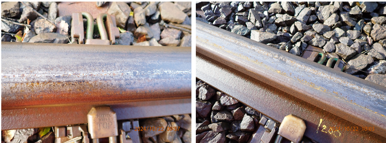
Figure 47: Example of visible contamination observed on the railhead on 22/10/2024 (the day after the accident) on the descending gradient at 100 metres (left) and 200 metres (right) before the collision location.
