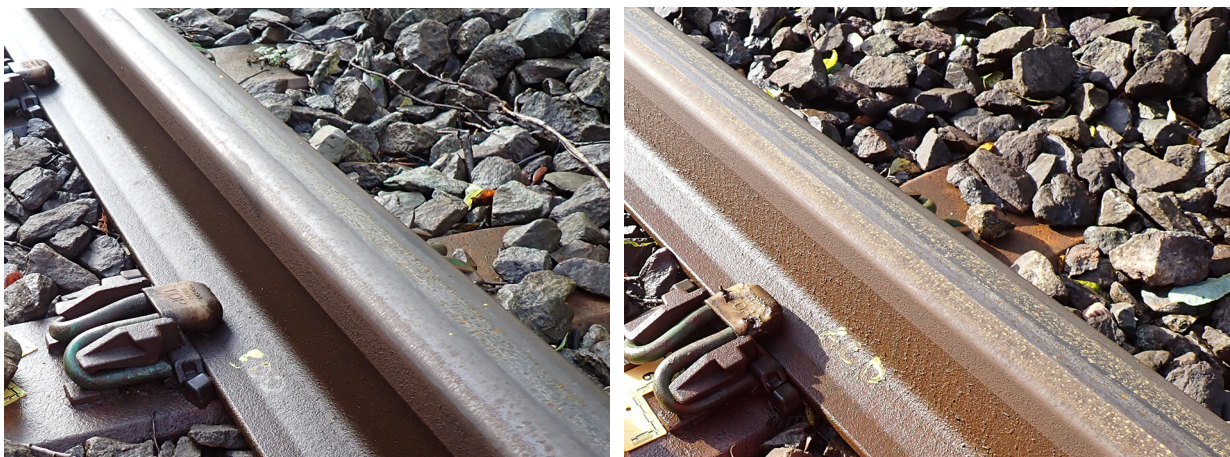
Figure 48: Example of visible contamination observed on the railhead, at around 10:20 on 22/10/2024 (the day after the accident), after the loop on the descending gradient at 500 metres (left) and 600 metres (right) before the collision location.
