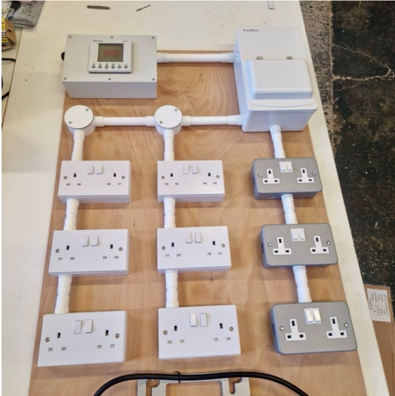
Figure 2: Instrumented laboratory rig using UK domestic socket circuits: (right) RCBO type AC protected ring-final; (centre and left) Spur B modern radial spur, RCBO type A protected. (© Arceio)
