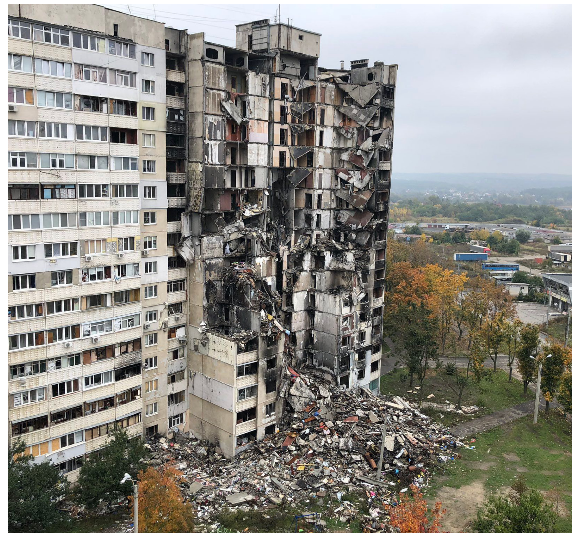
Damaged residential building in Kharkiv © Norman Foster Foundation
