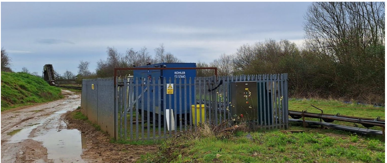
Figure 10 - Fairlop Site Diesel Generator and Conveyor Overview
