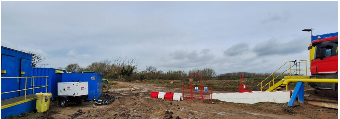
Figure 9 - Easthall Site 18 kVA Diesel Generator and Weighbridge
