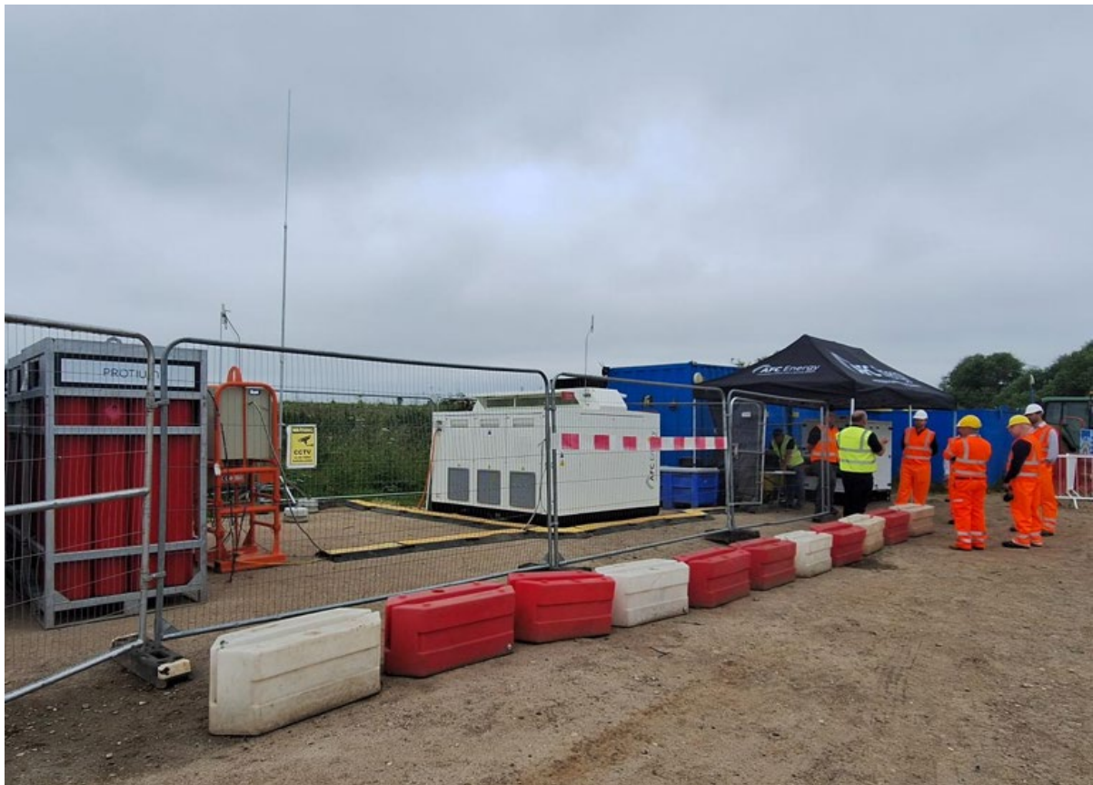
Figure 12 – Protium MCPs, AFC Energy’s 30 kW let-down station and fuel cell generator, and Energy Solutions’ BESS on Brett Aggregates site (left to right in images).
