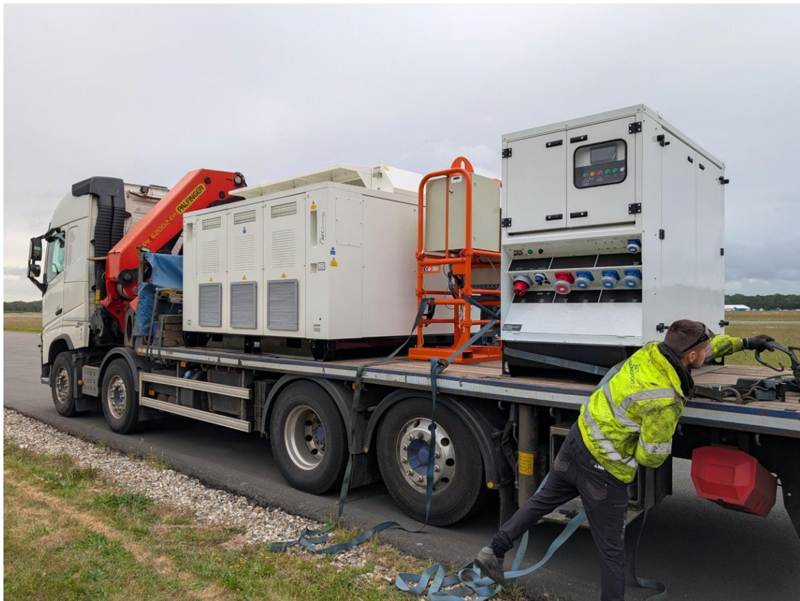
Figure 11 - AFC Energy's 30 kW fuel cell generator, let-down station, and Energy Solutions' BESS being readied for transit from AFC Energy to Brett Aggregates site (left to right in image).
