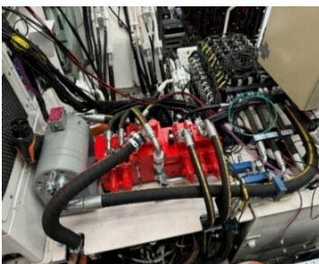
Figure 30: H-bridge valve setup for post-conversion data acquisition
