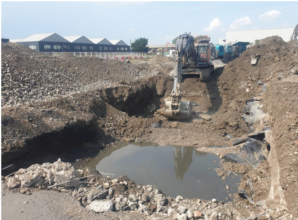
Photograph 1: Photograph taken during removal of the TBWRF attenuation tank by DSM, June 2023.
