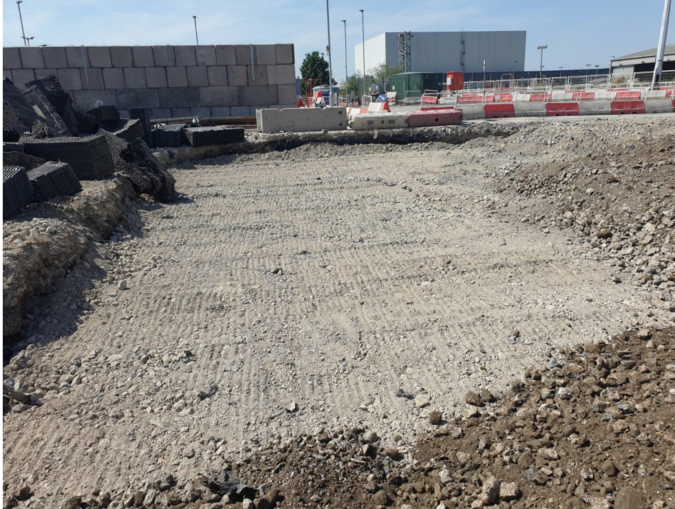
Photograph 2: The reinstated area following backfilling of the void left by attenuation tank removal, June 2023.
