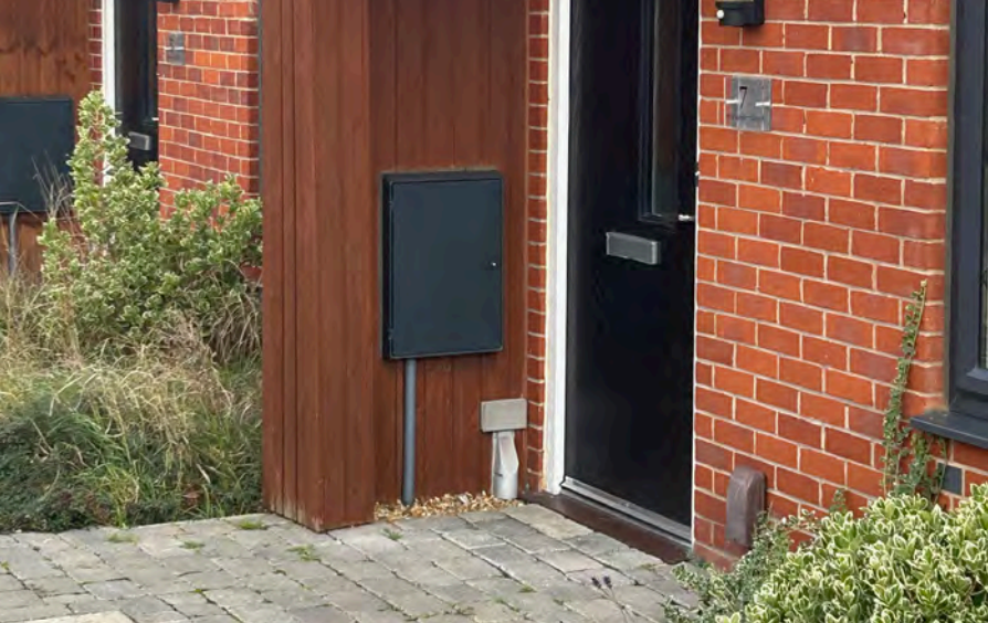
183 A utility box is better on a return wall or perpendicular to the front as it will be less visible, especially here tucked into a porch.
