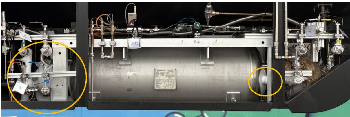
Figure 22 - Tank Ice Build
