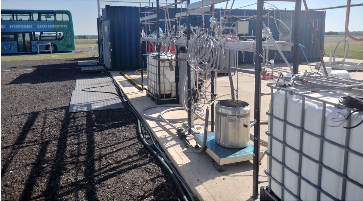
Figure 12 - Ground System Setup Build
