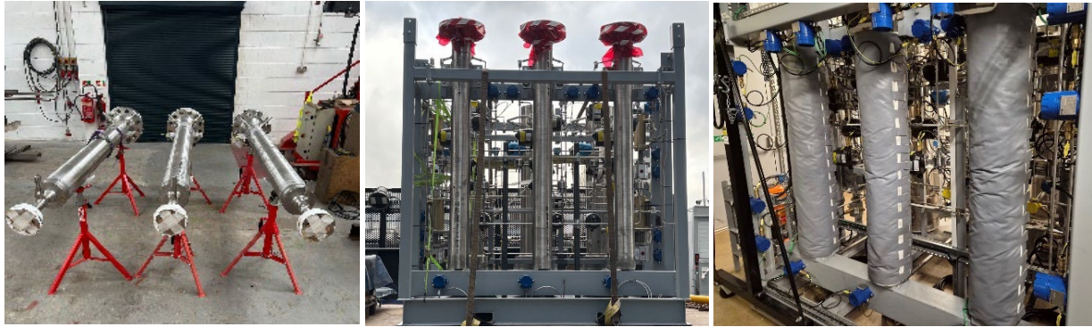
Figure 7: Chemical looping reactors from fabrication to installation in the plant (left to right)
