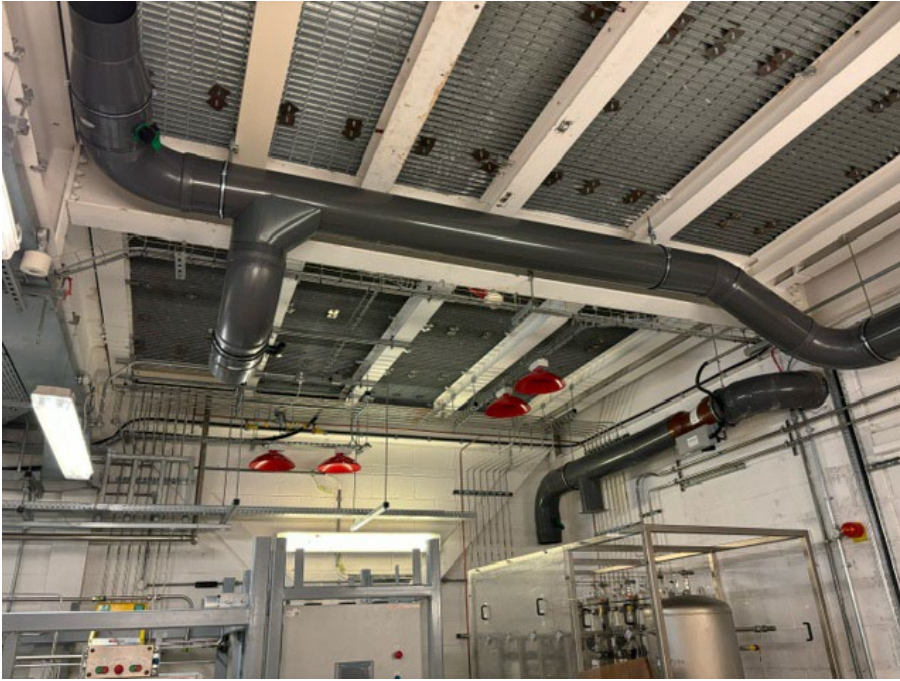
Figure 11: Extraction design and sensors installed in the RECYCLE plant site
