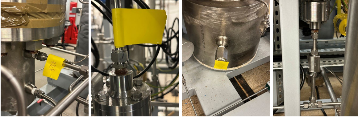
Figure 18: Examples of leak points identified during the pressure test carried out in the Syngas Generation and WGS-cooling system skids
