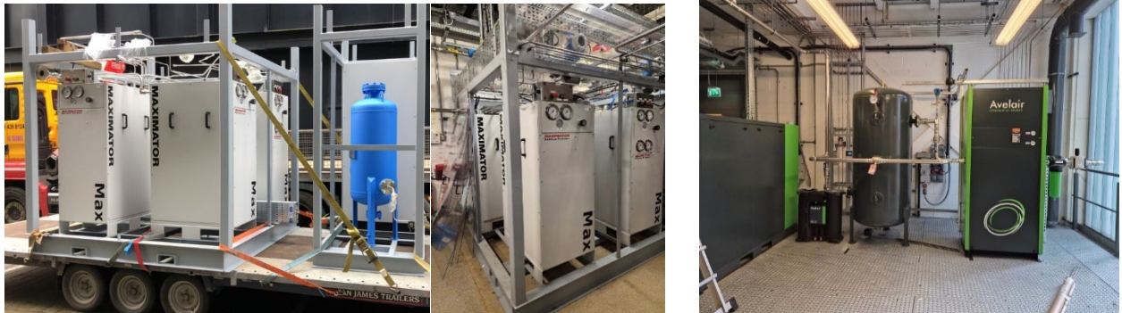
Figure 6: Gas booster skids and NG desulphuriser and right) Air Compressor(s)
