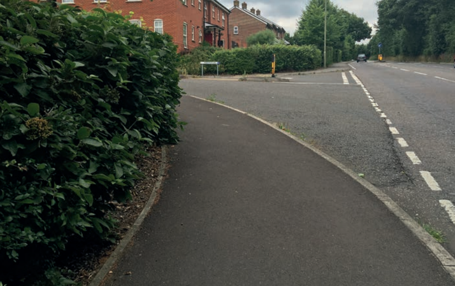
34 Overwide corner radii make it more difficult for pedestrians to cross the carriageway.
