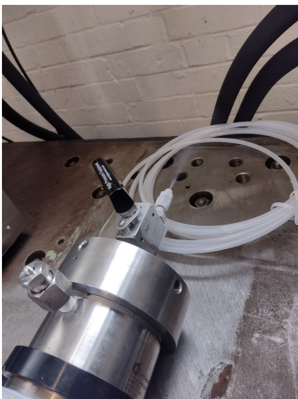
Frozen nozzle during local venting (test)
