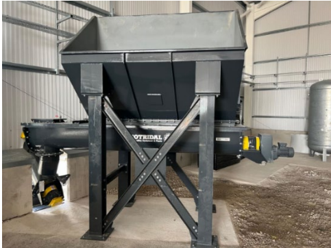
Figure 15 Feed hopper and feed screw/conveyor in place
