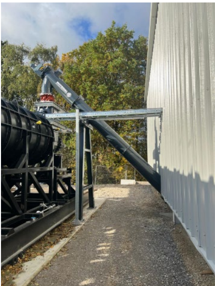
Figure 14 Feed hopper and feed screw/conveyor in place
