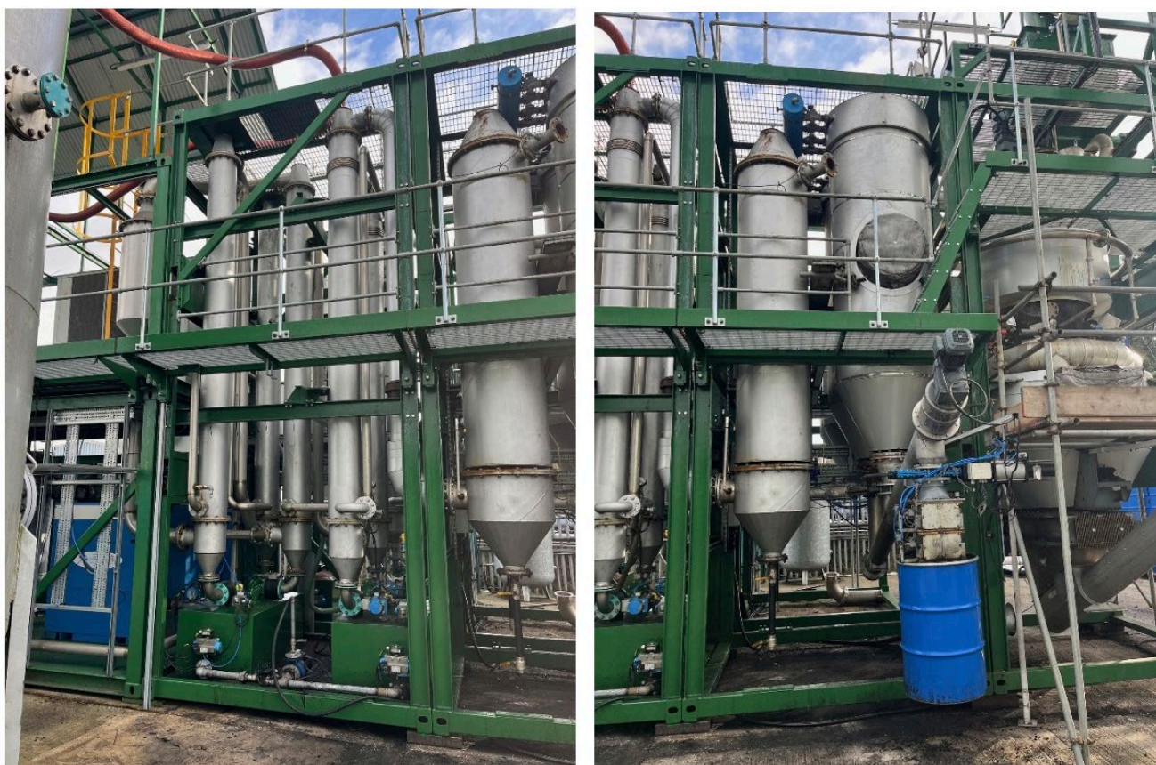
Figure 6 - Views showing hot gas filters (above blue drum in right-hand photo) and heat exchangers (middle of left-hand photo)
