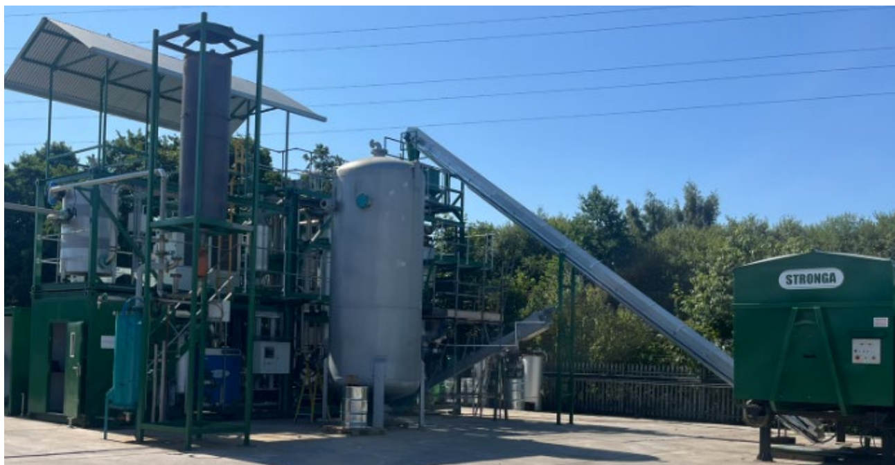
Figure 5 - A view of the front-end of the gasification process
