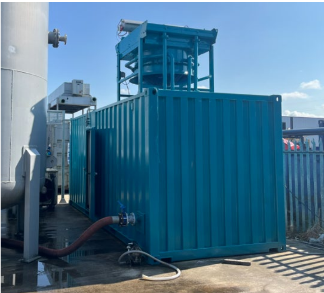
Figure 7 - View of the container in which the Gas Engine is positioned
