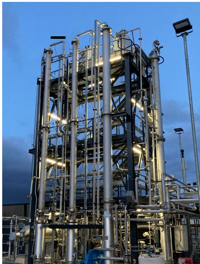
Figure 8: TERC CO 2 capture plant
