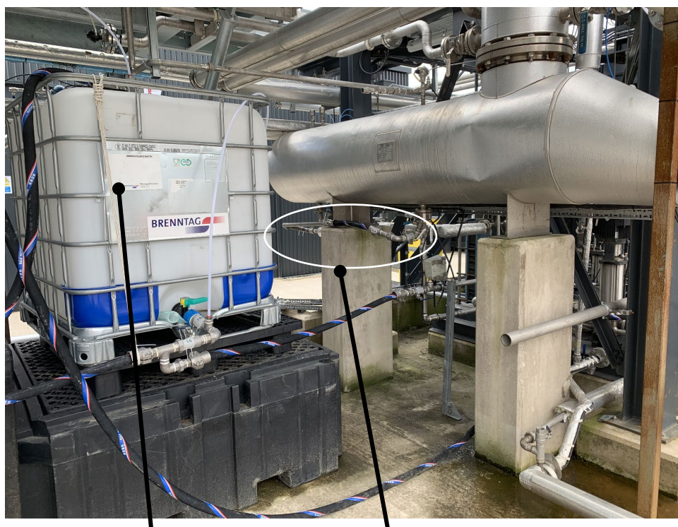
Figure 1.1 Lean solvent storage tank and reboiler weir bypass in place on TERC ACP
