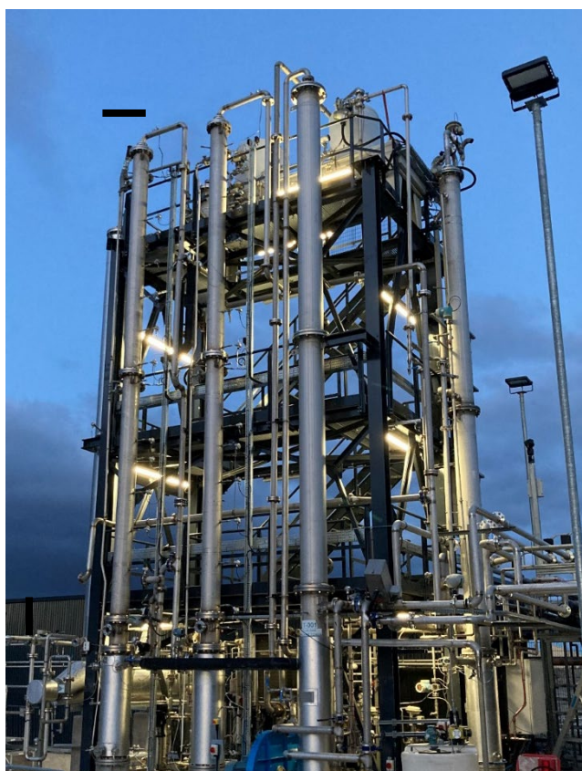
Figure 3.1: TERC CO 2 capture plant
