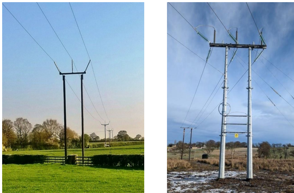
Figure 1: Types of overhead poles
