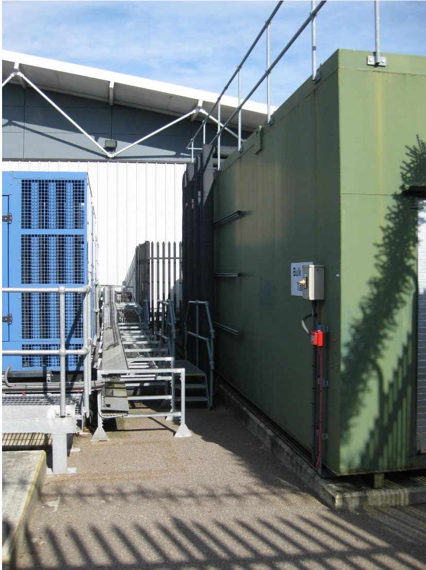
Photo C.2: Bulk Diesel Tank – front view
