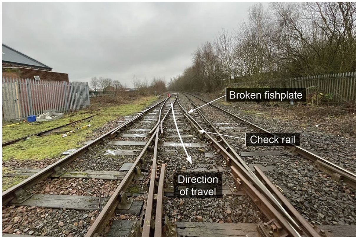
Damage to the crossover after the derailment.
