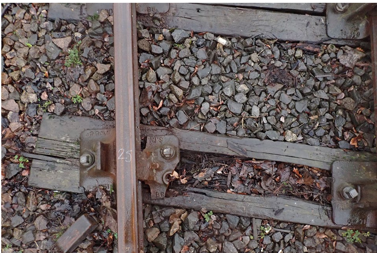
A timber sleeper inside the crossover after the derailment, showing rotten wood and insecure rail fastenings.
