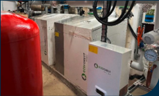
Image showing the heating equipment installed in the building's plant room. Courtesy of Oxford University Trinity College.
