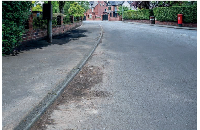
This image shows an urban road with significant accumulations of detritus. This means it is a grade D standard.
