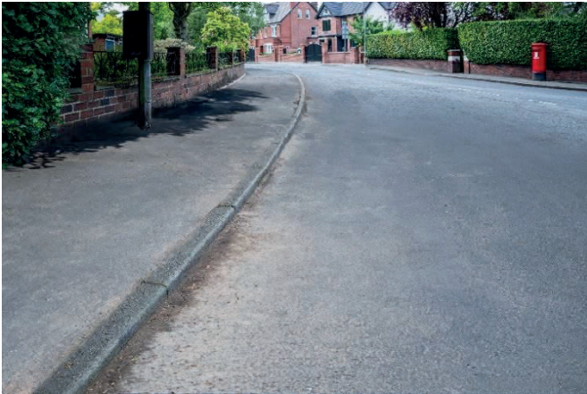
This image shows an urban road with widespread distribution of minor accumulations of detritus. This means it is a grade C standard.
