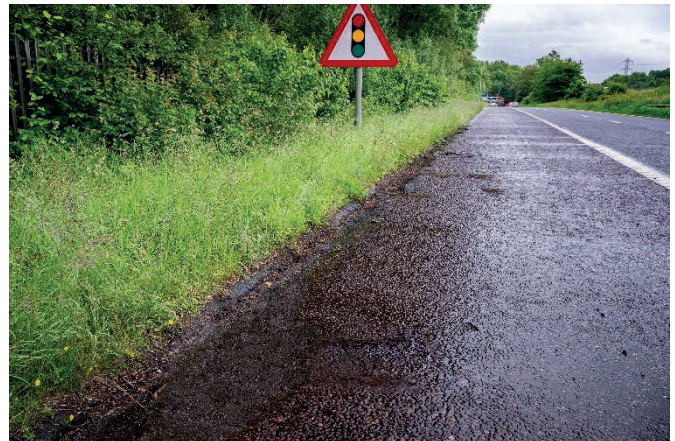
This image shows a major road with significant accumulations of detritus. This means it is a grade D standard.
