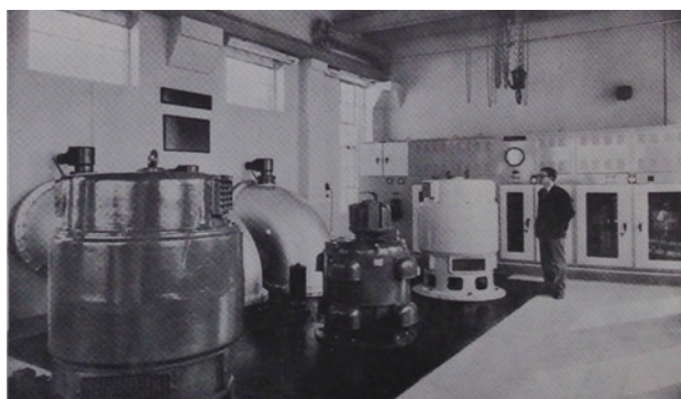
Interior of the newly built Adventurer's Pumping Station at Pode Hole in 1957 © Heritage South Holland.
