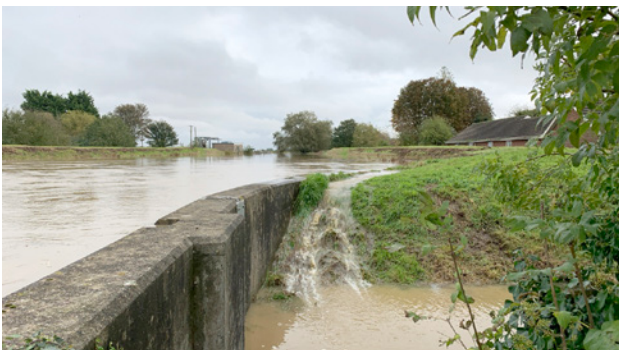
Overtopping of the Wainfleet Relief Channel in October 2023. The relative water level compared to the property visible on the right shows how critical these embankments are © Environment Agency
