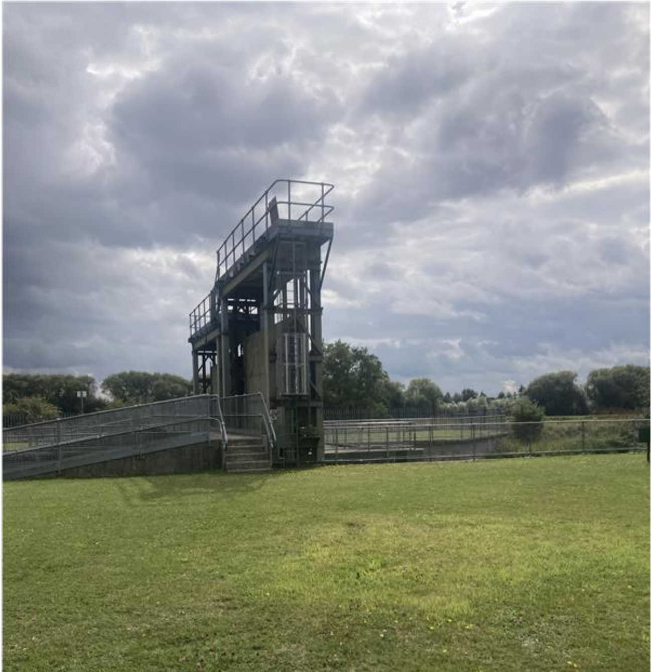
Figure 15: One of the two sluice gates at Hockwold looking South (upstream) (© Arup 2024)
