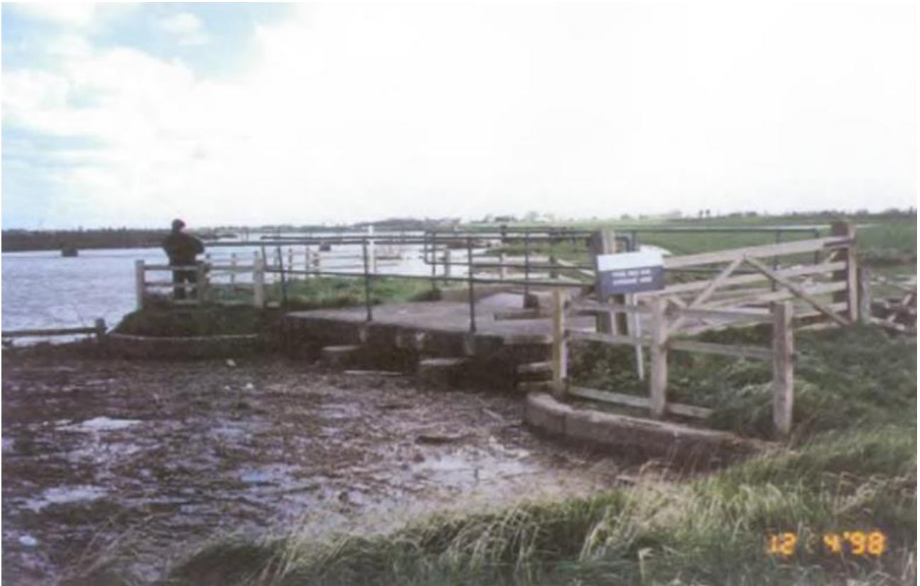
Figure 20: Four Mile Bar Siphon not fully primed during the 1998 flooding event Environment Agency
