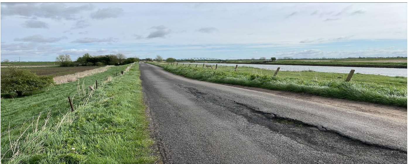
Figure 10: Photo of the Deeping High Bank, the Cradge Bank can be seen on the far side of the Welland. The pavement in the high bank is subject to deep rutting and deformation
